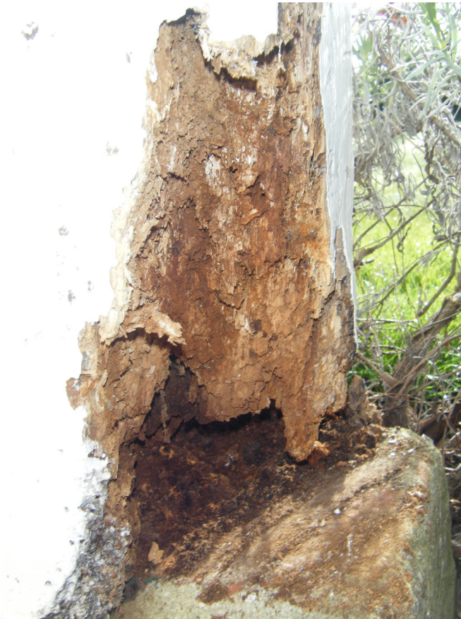
Cement damage to a structural timber frame
