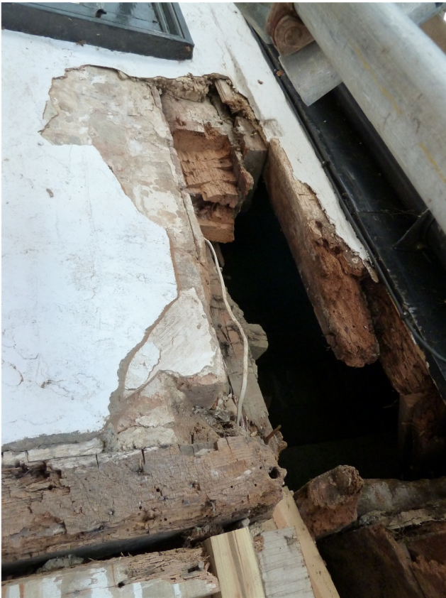
Damp damage caused by a cement render
