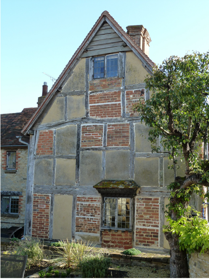
Damage by a cement render
